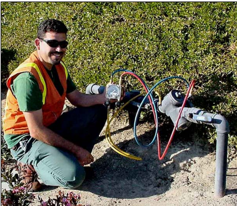
Tom Sanchez tests reduced pressure backflow prevention device.
